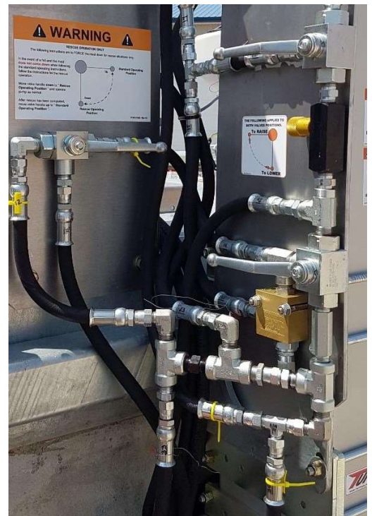
Figure 13b, Warning / Operation Labels located on Mast
