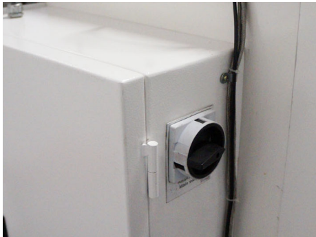
interruptor principal bloqueable
